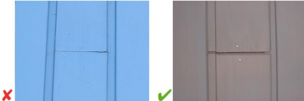
Figure 8 - Butt joints incorrectly installed (Source: Centrum Hout, 2024)
